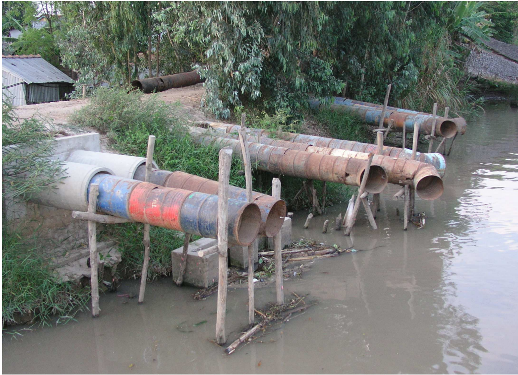
Figure 41 Pipes between a canal and a high dike compartment
