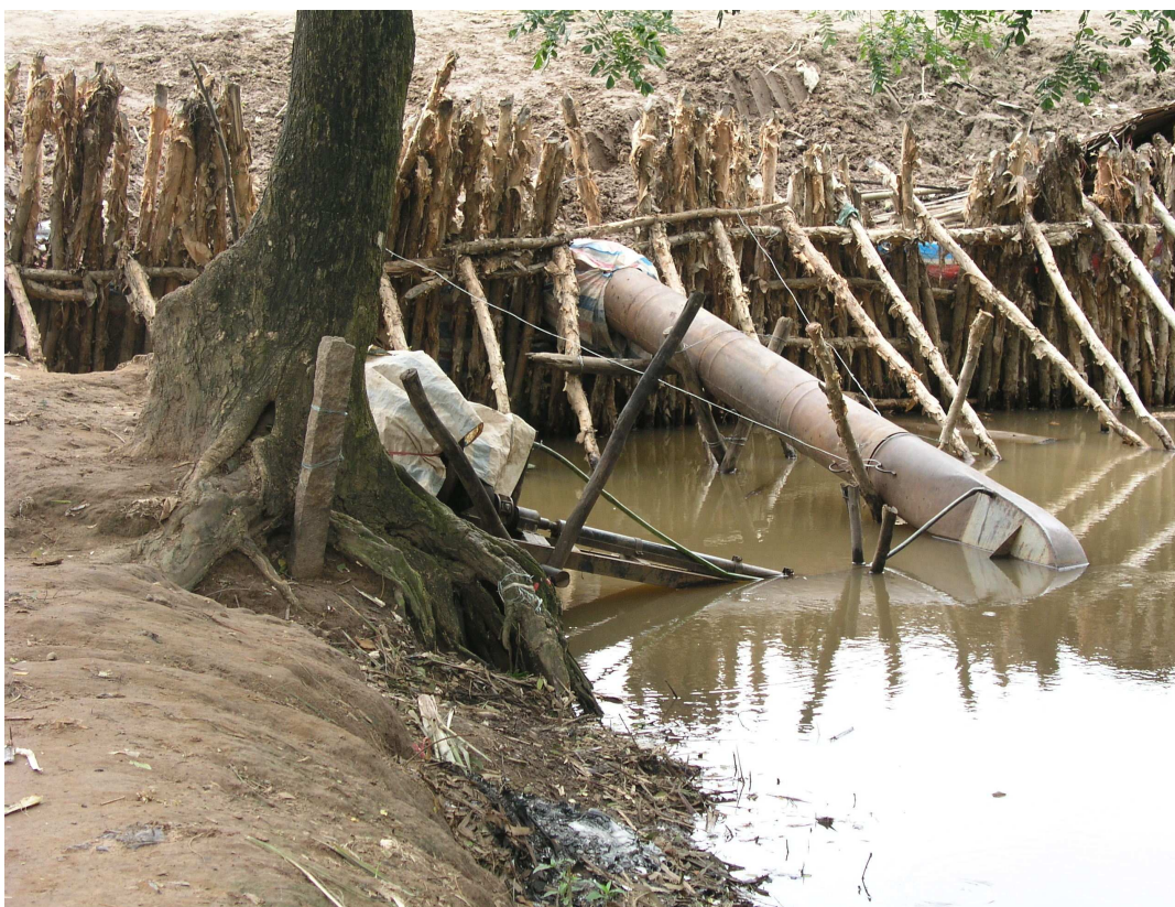
Figure 59 The recently completed high dike wall in Binh Thanh Commune after the first flood season
