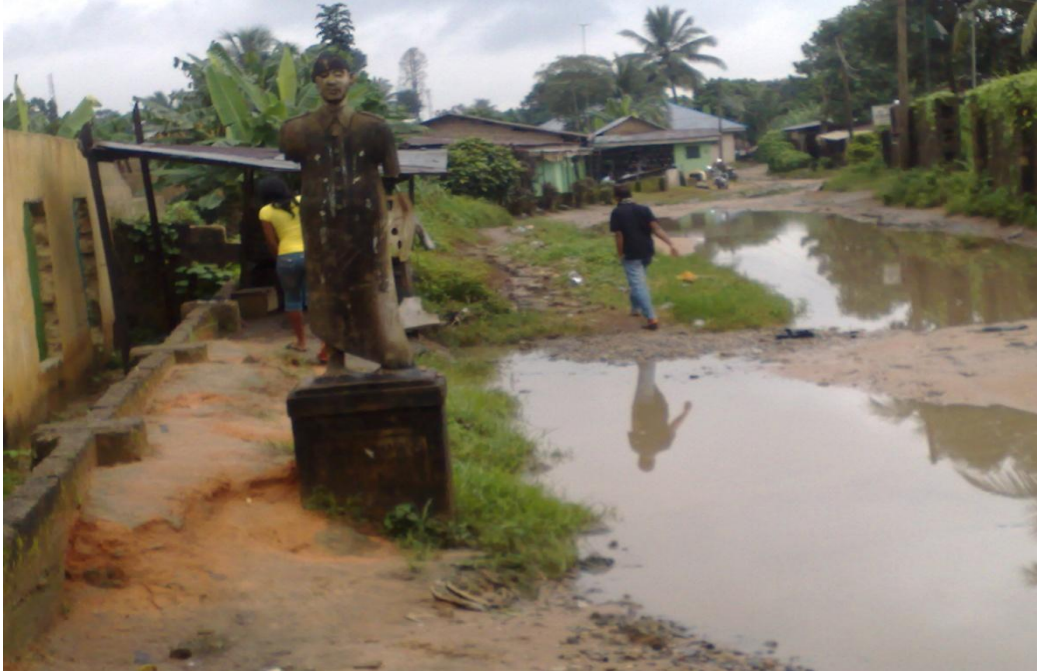
FIGURE 4.16: Flooded Road in Uyo where cars drive through.
